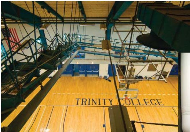
View from the mechanical room—"above the rim." Catwalk shown descending is the only access
