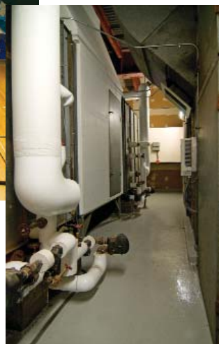
Revitalized mechanical room high above the gym floor
