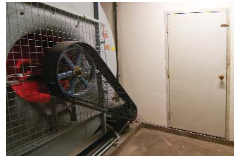
One of four large fans. The full size door was the size of the access to the mechanical room without demolition
